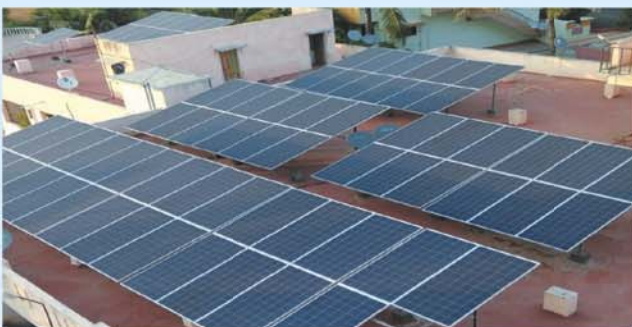
G- Energy Project Photograph (System 25 KM)
