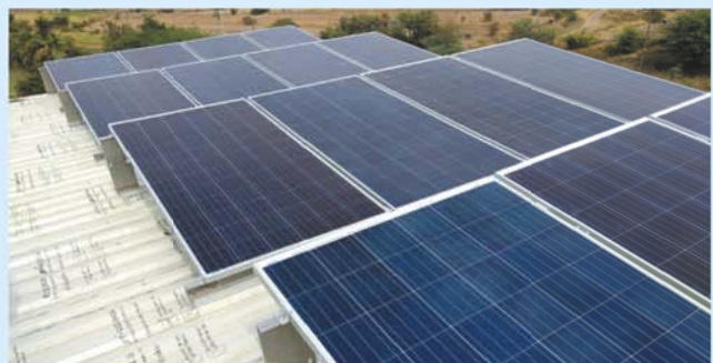
G- Energy Project Photograph (System 10 KM)
